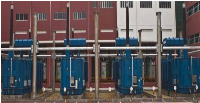
China | EETI 750kV Power Transformer
