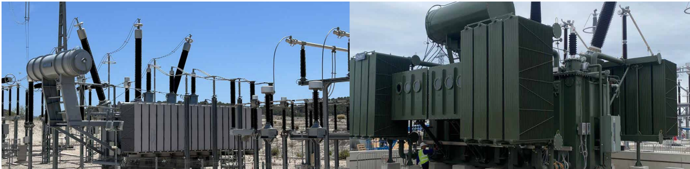
Spain | Renewable Energy EPC Project 400kV 400MVA Power Transformer
